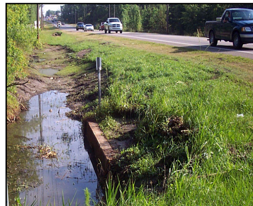
Pictured is a ditch and drainage structure near Cascade Drive and Capital Circle Southwest. The view is facing north.
